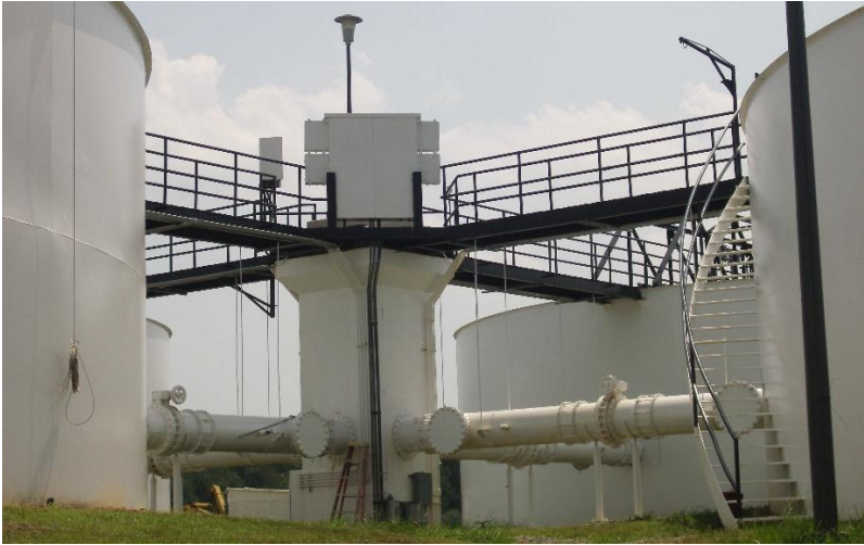
Clarifiers at the water treatment plant help remove solids from untreated water which improves turbidity and water quality.
