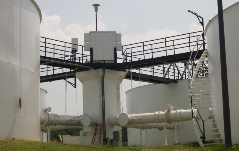
Clarifiers at the water treatment plant help remove solids from untreated water which improves turbidity and water quality.
