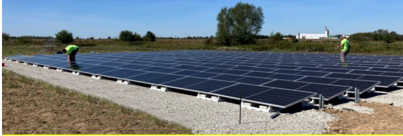
Figure 2.5: EXAMPLE (Ground View): SIMILAR PROJECT Completed by Tick Tock Energy. 86 kW (DC) Installation for Village of Dieterich Waste Water Plant
