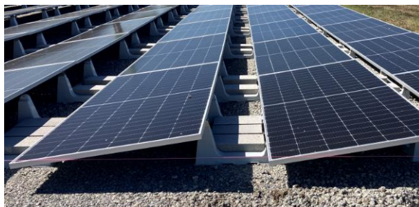
Figure 2.4: Example Close-Up View of Low-Profile, Ballasted Ground Mount Solar Array
