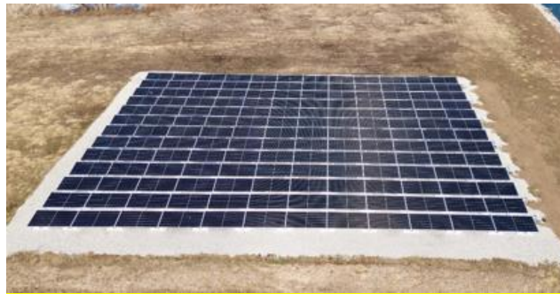
Figure 2.6: EXAMPLE (Aerial View): SIMILAR PROJECT Completed by Tick Tock Energy. 86 kW (DC) Installation for Village of Dieterich Waste Water Plant
